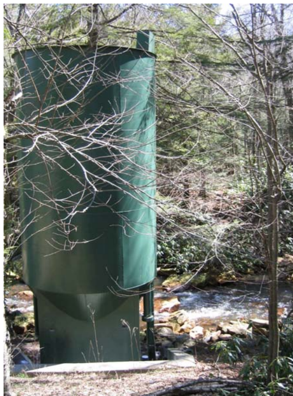
Cherry Creek lime doser located in a steep mountain valley.
